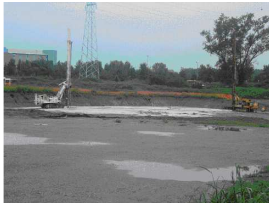
Figure 1.15: The CNAO site at the end of August 2005. Jet-grouting techniques are adopted to realize the foundations of the building.
