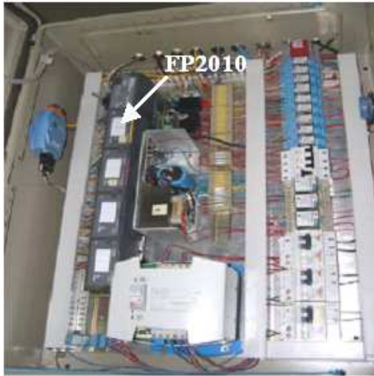
Figure 4.25: Electrical panel for the SLIM beam monitor.
