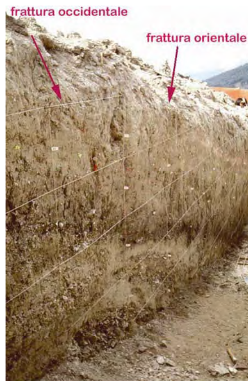
Figure 4.11. Picture of Trench 1 south wall, the two red arrows delimitate the main fracture zone internally totally disrupted in terms of sedimentary structures.
