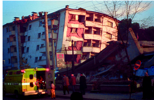
FIG. 1. Tilted building after the Izmit Earthquake, Aug 17th, 1999, Adapazari village, Turkey. Picture: Courtesy of Mustapha Meghraoui, IPGS.
