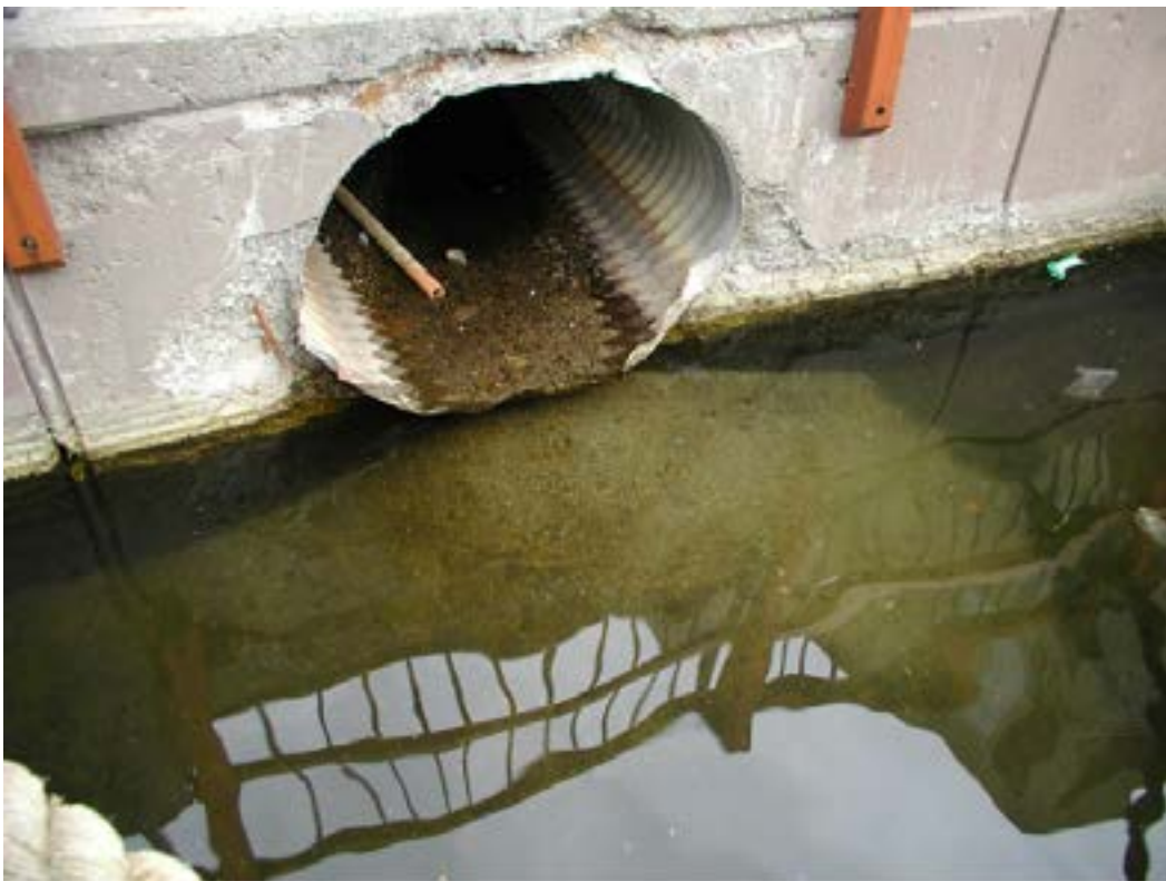
Figure 1: Bedload sediment accumulation in sewerage and near inlet to pond (Snowmass, CO)
