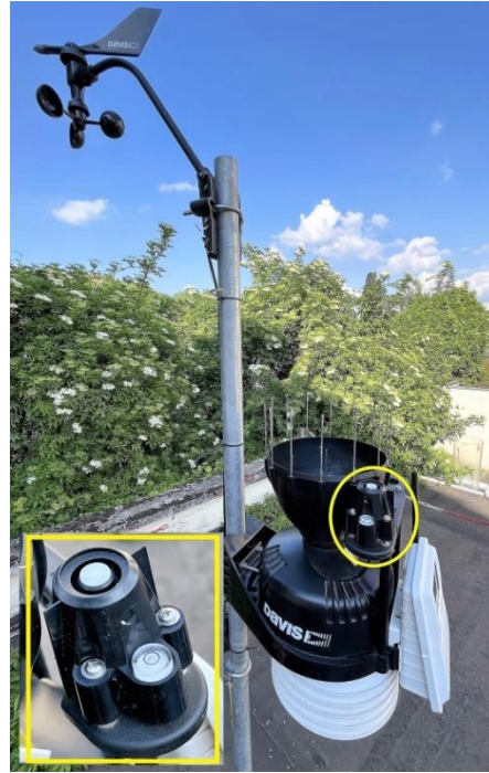
Figure 7-13: The installed weather station. The solar pyranometer is marked with yellow and zoomed.
